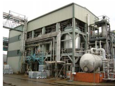
a hydrogenation plant
