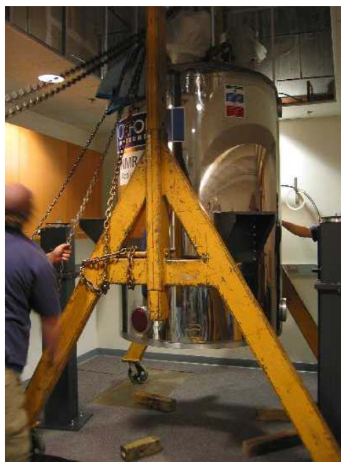
Installation of 16.45 T magnet in Hasselmo Hall.
